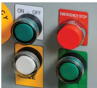
Control Panel Labels
