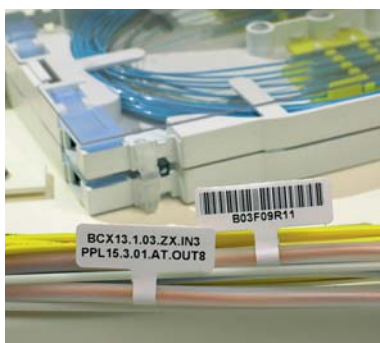
Fibre Optic Cable Markers
